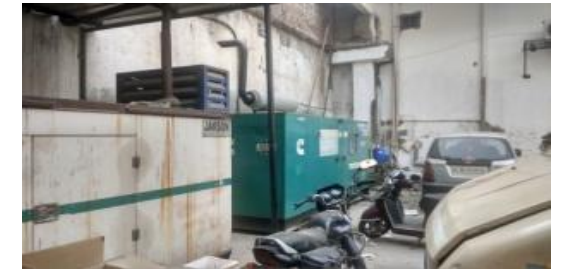
Power back up
